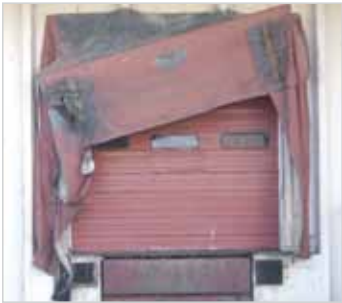
Damaged Loading Dock Shelter
