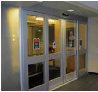
Automatic Sliding Door After
